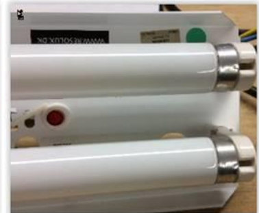
c. Power on L1 only (not work)
